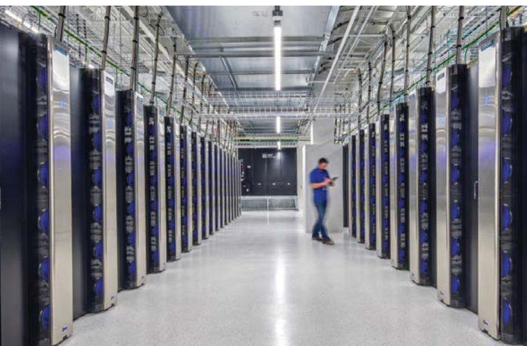
IMCO's Infrastructure portfolio: State-of-the-art, enterprise grade data centre located in downtown Atlanta, Georgia. Images by DataBank.
