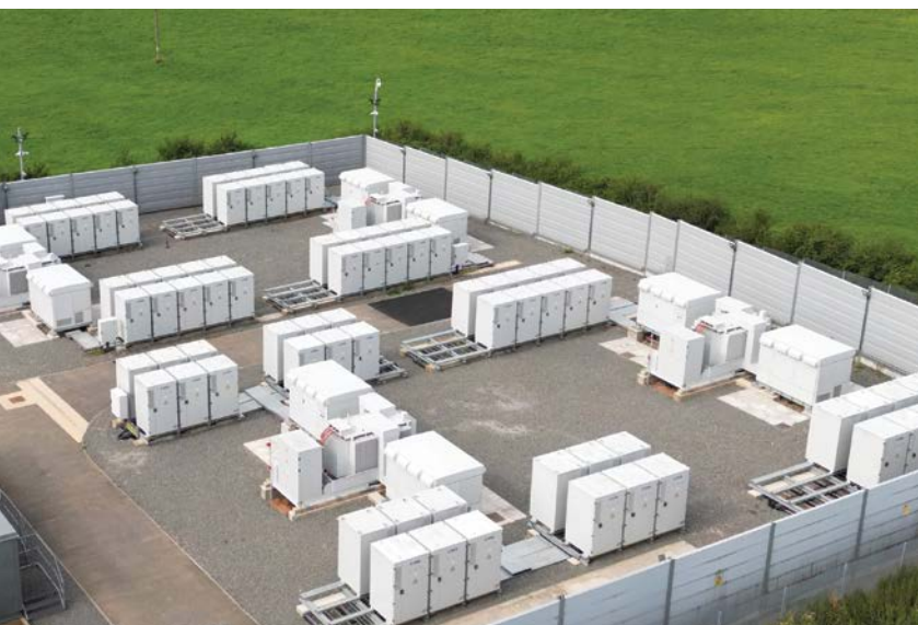
Pulse Clean Energy's Willoughby battery storage site in the United Kingdom. Image by Pulse Clean Energy.
